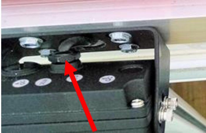
Damaged Seal & Using Center Hole
